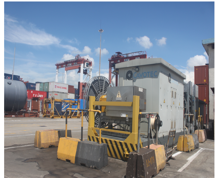
Shore power infrastructure in Shekou, Shenzhen
